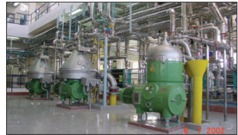
(i) A piping network in an industrial facility.
